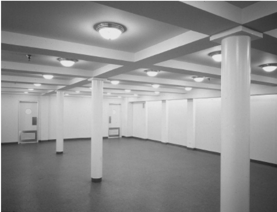
Figure 12.58 Ceiling-mounted diffuser luminaires.
