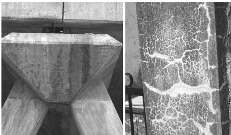
Fig. 4.15 Cracking caused by alkali-silica reactions
