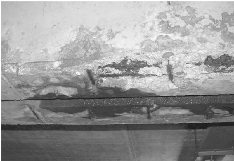
Fig. 4.14 Concrete degradation due to corrosion of reinforcements
