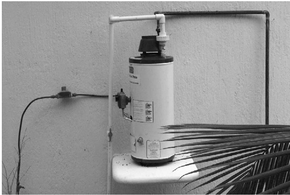
Figure 4.6.8 Small on-demand hot water heater.
