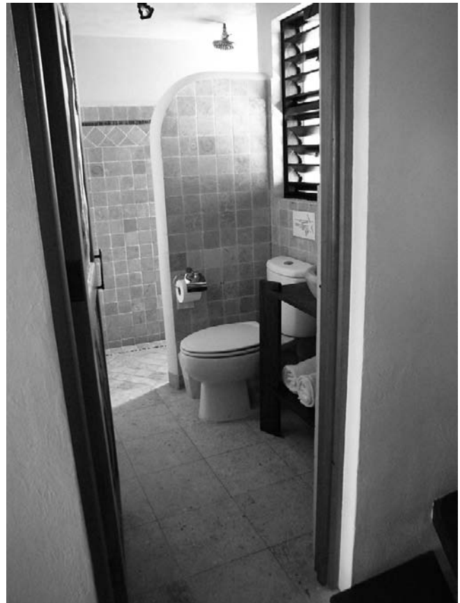
Figure 4.5.7 Standard dual flush toilets generate enough liquid waste for the created wetland to be viable.
