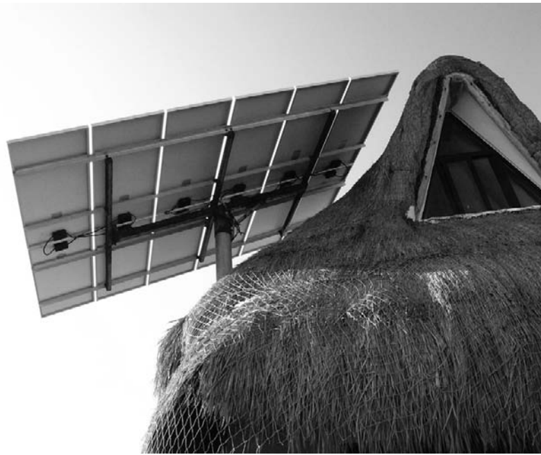
Figure 4.5.6 The principal source of power is a set of 20 photovoltaic panels above the roofs of guest units.
