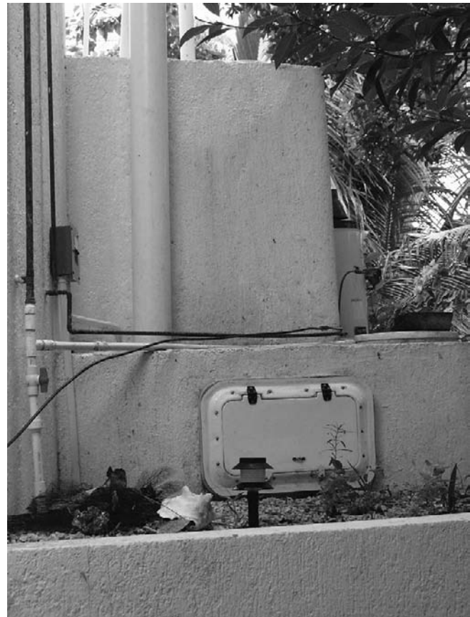
Figure 4.6.10 Each building has its own composting toilet unit.
