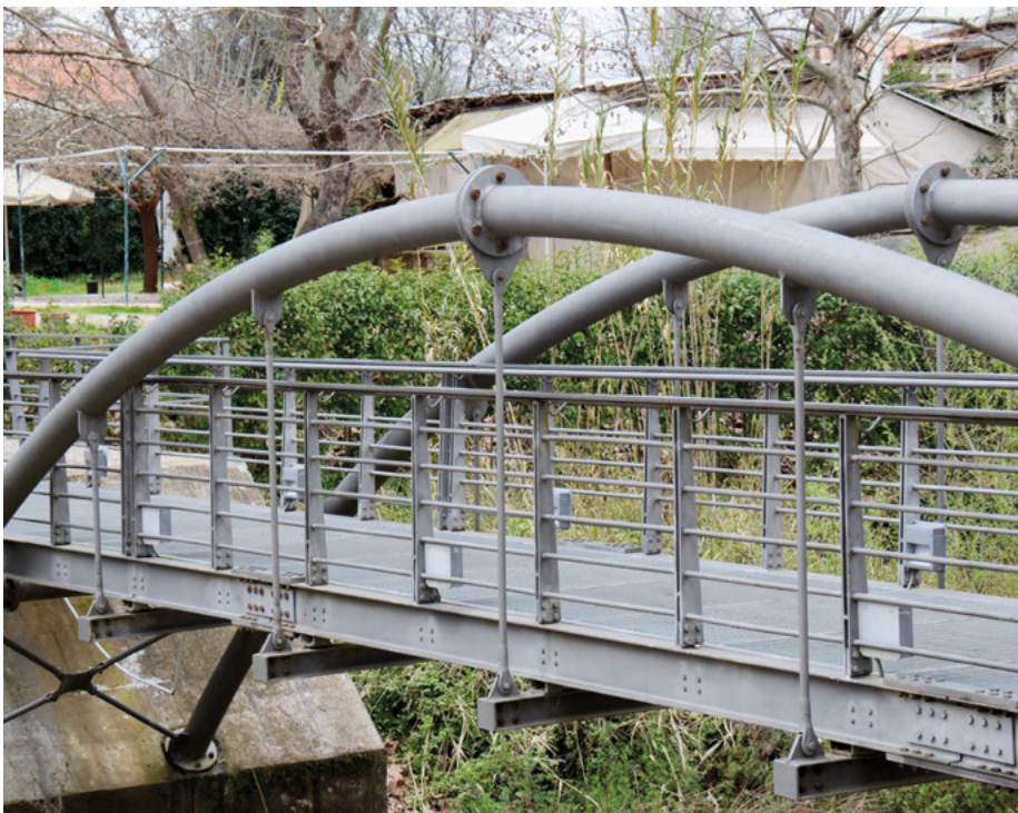
This pedestrian bridge in Olympia, Greece, uses durable galvanized steel for its structural and railing components. Yet some of the bolts appear to be plain carbon steel and are oxidizing. This is easily avoided by specification of galvanized fasteners.
