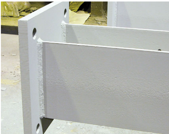
Steel has slight surface imperfections and roughness as a result of its manufacturing process. While this might be acceptable in AEES 1 steel (as discussed above), it must be remediated for AEES 4 material.
