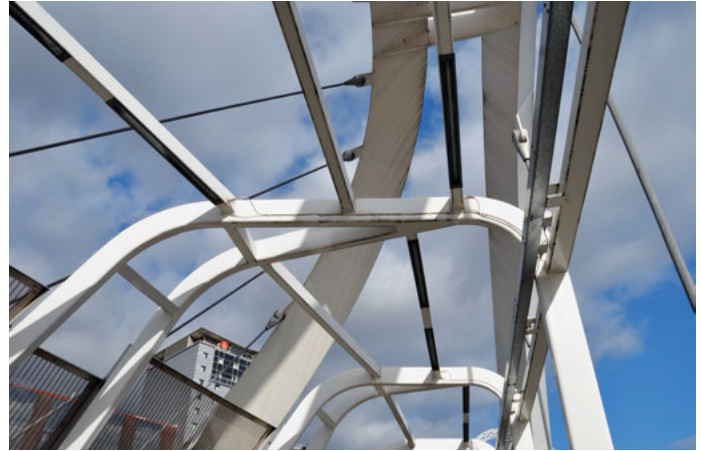
The exterior structure of Wembley Stadium in London, England, designed by Foster + Partners, shows evidence of dirt build-up due to rainwater runoff on the underside of the steel frame.
